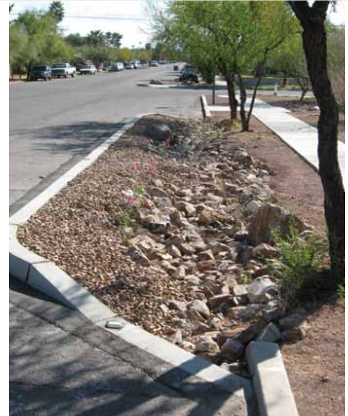
In this just-installed chicane, 4"-8" rip-rap is used in the channel where stormwater will flow rapidly, and 1" gravel covers upslope areas.
