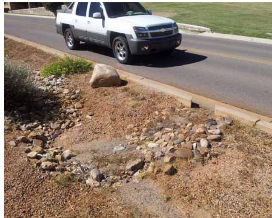
Simple, angled curb cut enhances capture of stormwater moving along the gutter.
