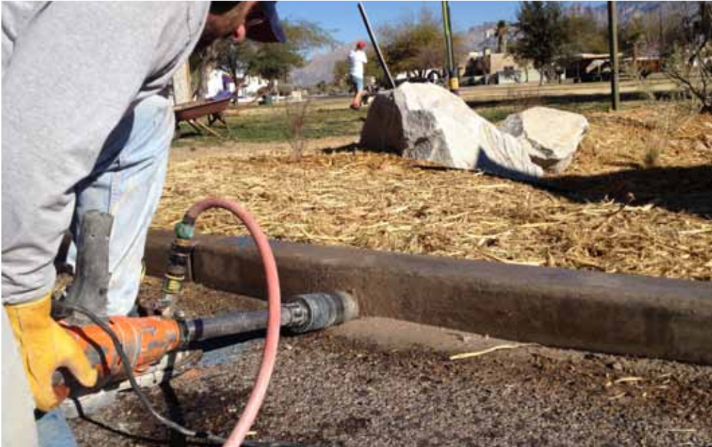
Drilling a 4" core at a slight downward angle to enhance water flow into basin.
