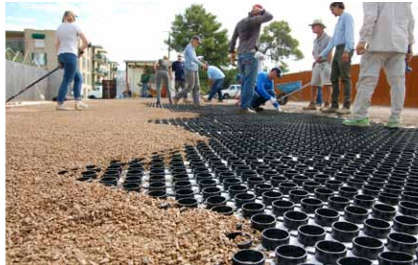
Participants in a professional green infrastructure training learn how to install a permeable parking surface. A recycled plastic base retains a gravel surface that promotes infiltration.
