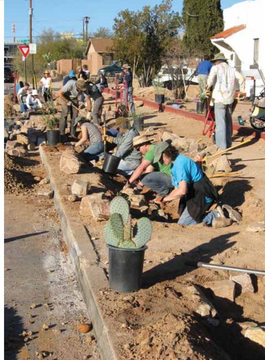
Volunteers install bioretention basins in the right-of-way at a workshop in Tucson led by Watershed Management Group.
