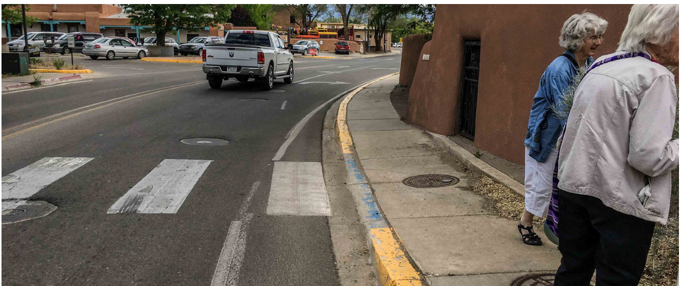
Narrow and deteriorating sidewalk in the MRA District. Courtesy of Jim O'Donnell
