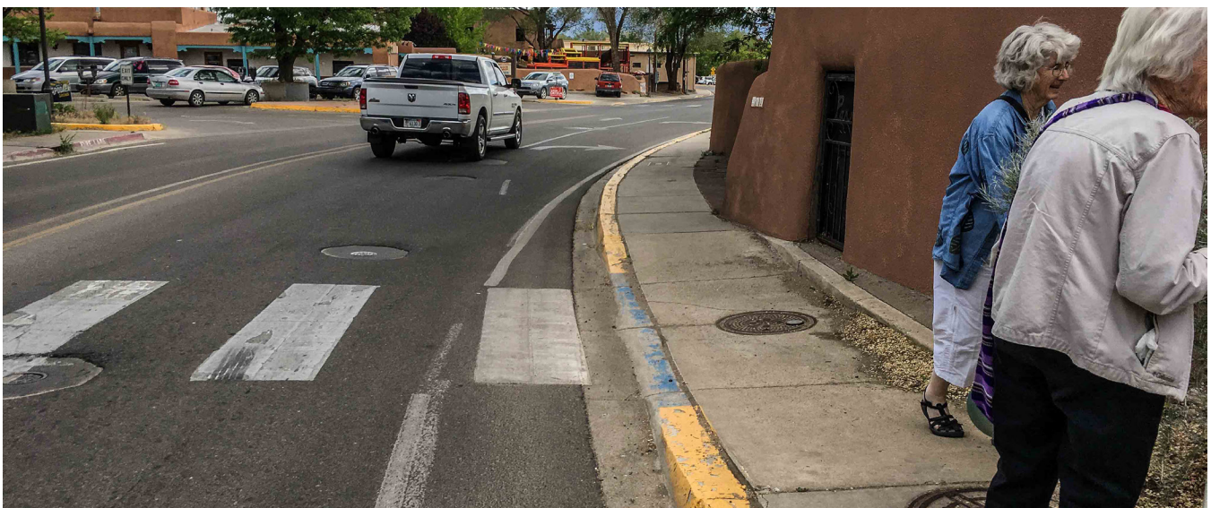
Narrow and deteriorating sidewalk in the MRA District. Courtesy of Jim O'Donnell
